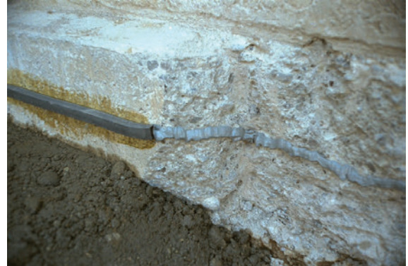
Rough Concrete Cold Joint
